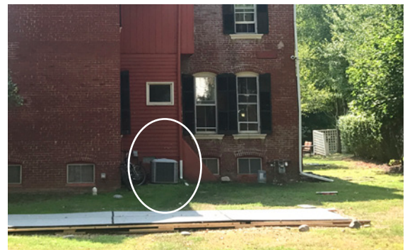
Mechanical units and generators should be placed on the rear façade, even if they are visible from secondary alleys.
