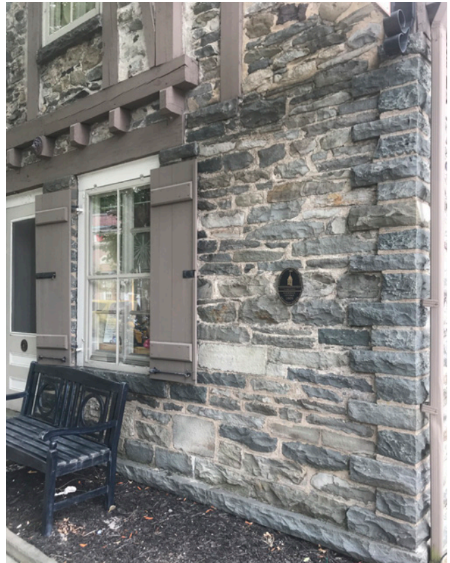
Bluestone is a distinctive local material that should be retained and preserved. Rough ashlar masonry, irregular sizes and coursing, and quoining at building corners are typical character-defining features.
