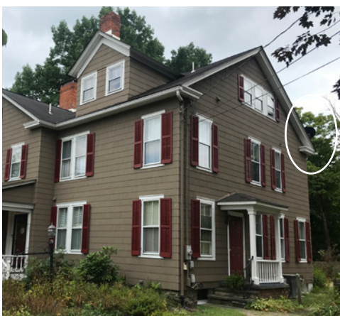
Satellite dishes on rear roof slopes can be almost entirely concealed from the public right-of-way.
