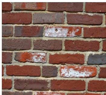
Efflorescence is a white haze caused by the migration of salts through masonry units.
