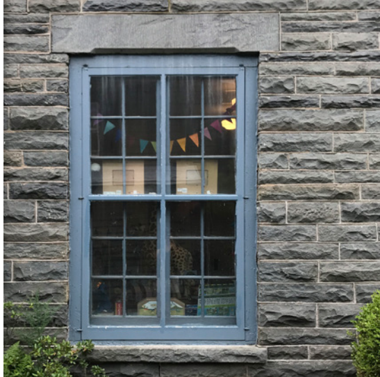
An example of a historic multi-lite wood window and wood storm window.
