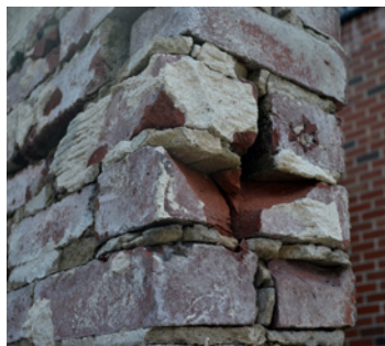
Mortar is incompatible with historic masonry when it is too hard and causes brick spalling and breakage.
