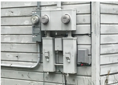
Grouping meters on a secondary façade and painting reduces the immediate visual impact.
