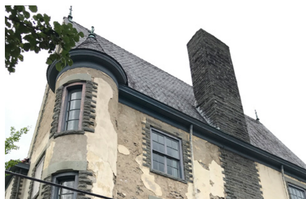
Chimneys with decorative brickwork or stonework are distinctive and should be preserved.
