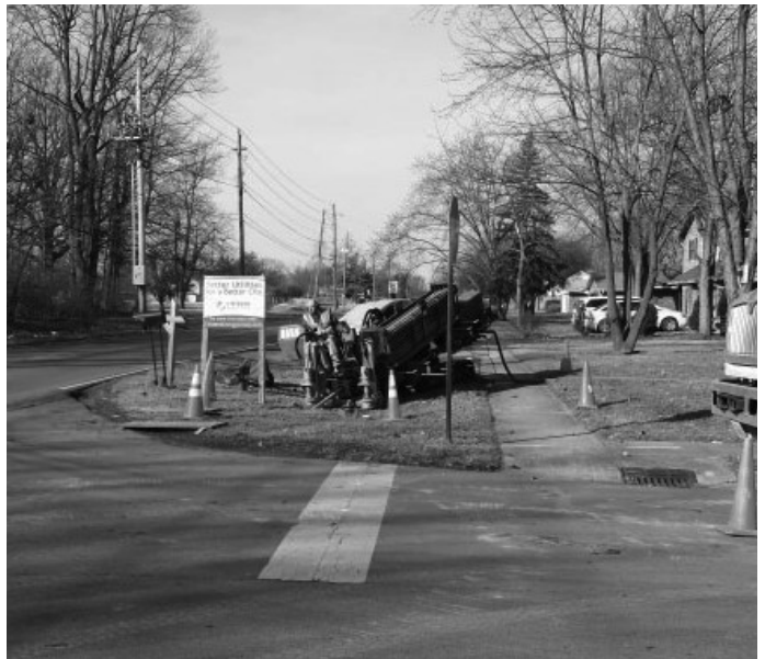
Above: Directional boring machines allow pipe to be installed under streets without disruptive street cutting and excavation.
